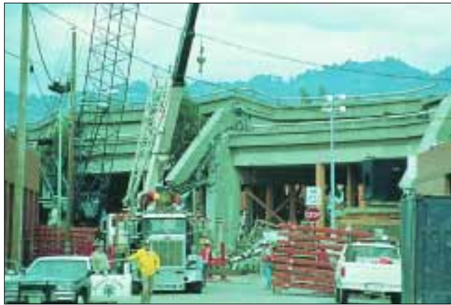
◆ FIGURE 4.26 The I-880 freeway failed because it was built on bay muds that reacted to seismic waves like a bowl of gelatin. Pictured is the Cypress Street viaduct with the upper deck collapsed upon the lower one. There was loss of life here.
